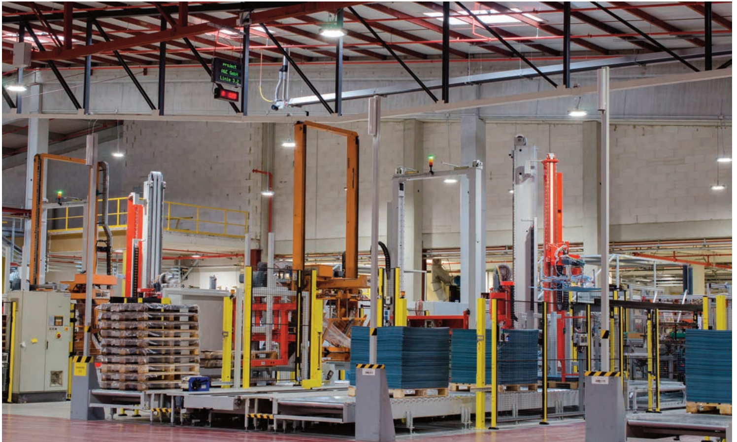
The LED lighting now delivers 190-250 lux at floor level.
